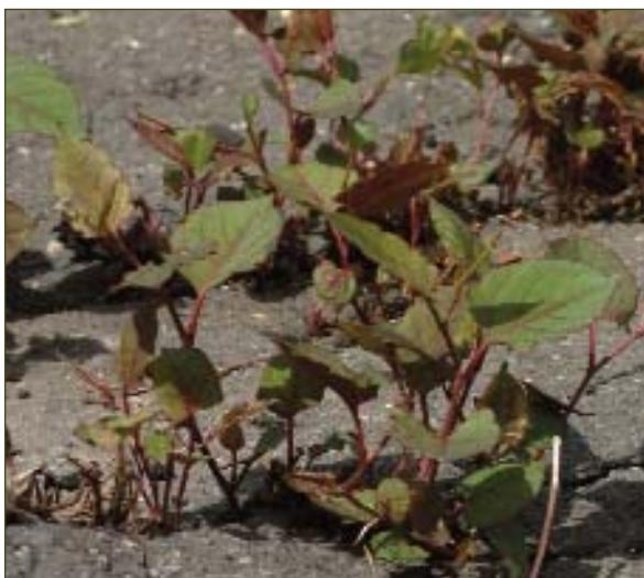
Figure 1: Japanese Knotweed breaking through a paved surface (Photo: Mike Dodd)
